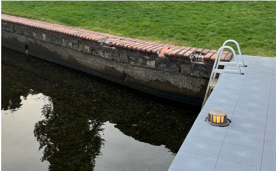
Photo of existing failing masonry bulkhead cap
